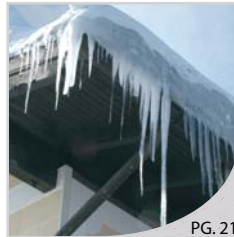
Roof & Gutter De-Icing
